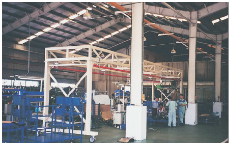
▲ Mobile Gantry Crane
